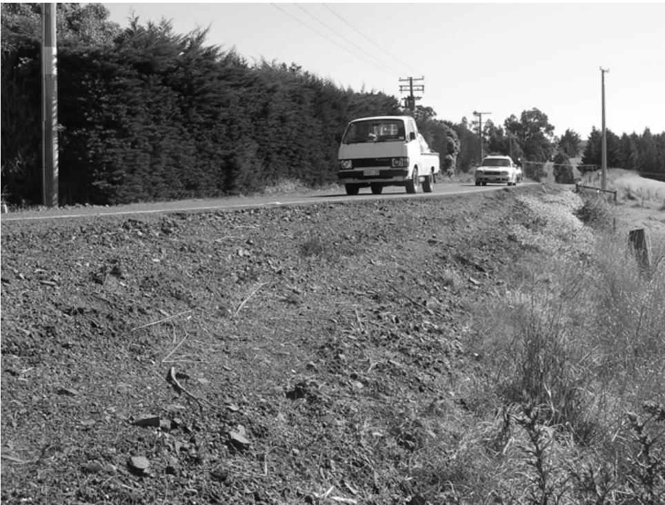
Figure 3: An example of the narrow verge and very steep unstable slope which face would be walkers between Waldronville and Green Island.
